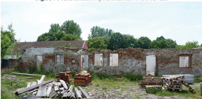
Figure 9 Found condition of the small Hornwerk barrack
